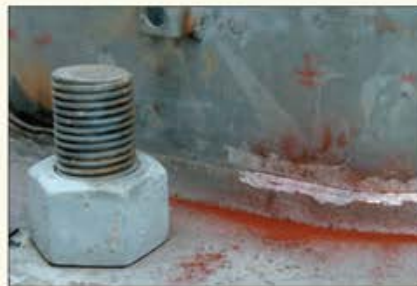
An ASNT inspector ultrasonically tests a base-weld connection. In the last frame, the defect is revealed at the toe of the weld on the pole bend line.
