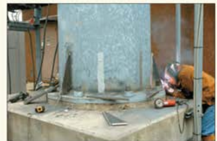
Installation, by a certified welder, of reinforcing base-plate stiffeners to strengthen the base plate.
